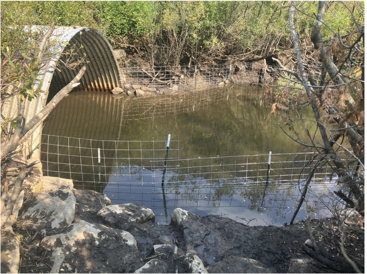
Culvert – Beaver Coexistence
