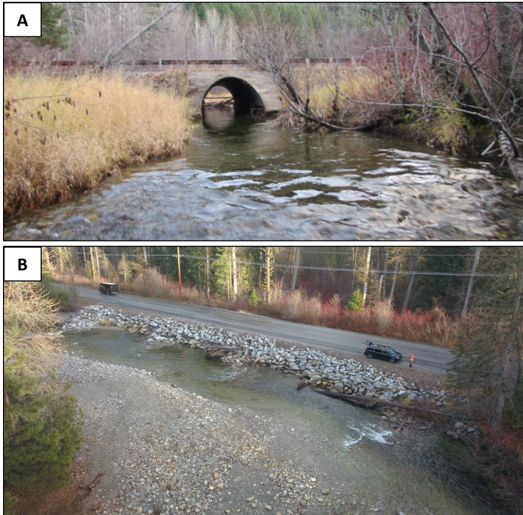
Figure 3. Infrastructure within the project area includes (A) CMP culvert with concrete headwalls (RM 3.75) which provide connectivity to the side channel on the east side of the highway, and (B) Highway 207 (RM 4.4) which has been reinforced with rock in several locations and can be removed with highway relocation and allow hydrologic connection to historic floodplain areas.
