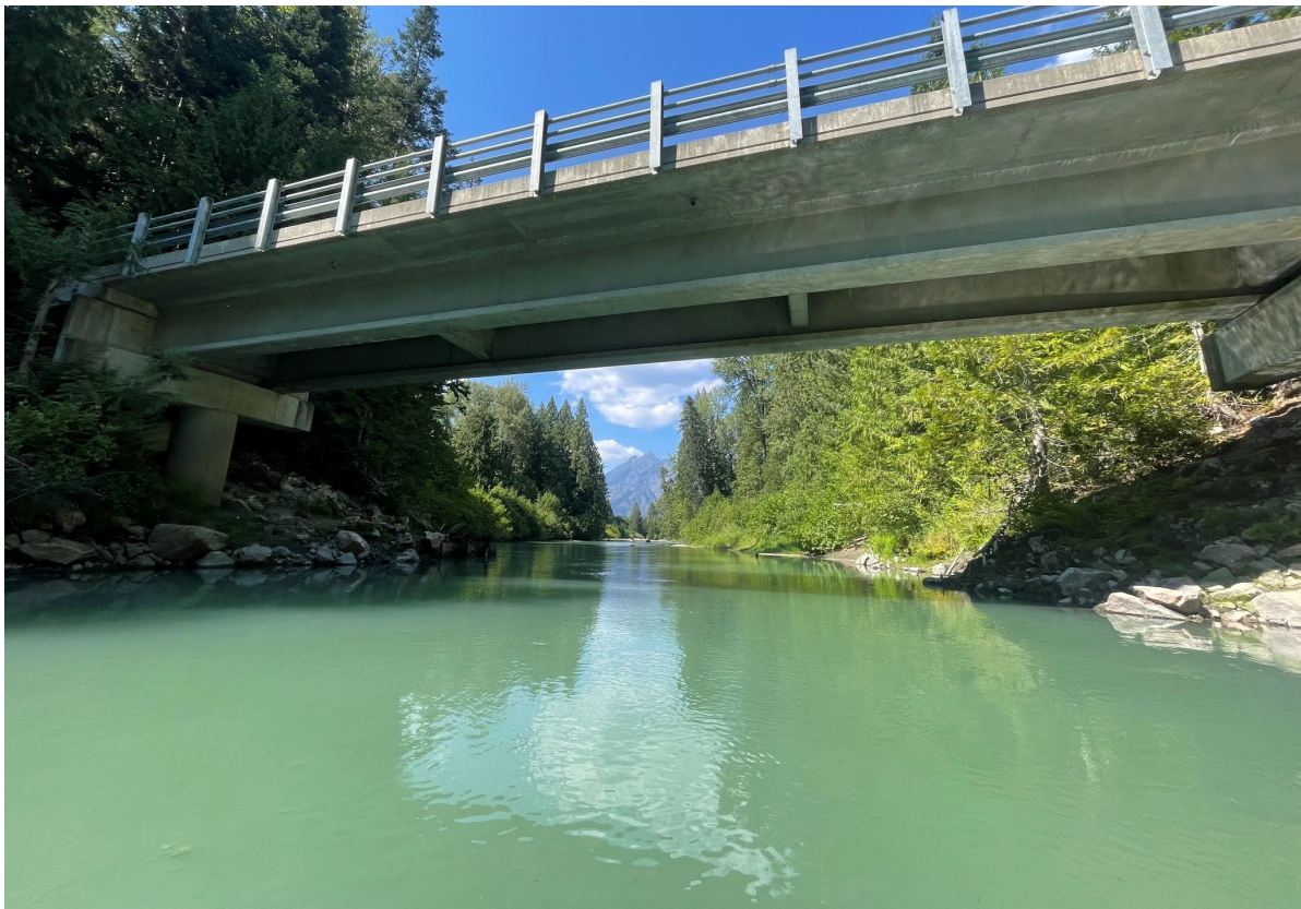
Figure 8. Photo of riprap protecting the Sears Creek Bridge around RM 7 (at the break of Reach 4 and Reach 5) on the mainstem of the White River.
