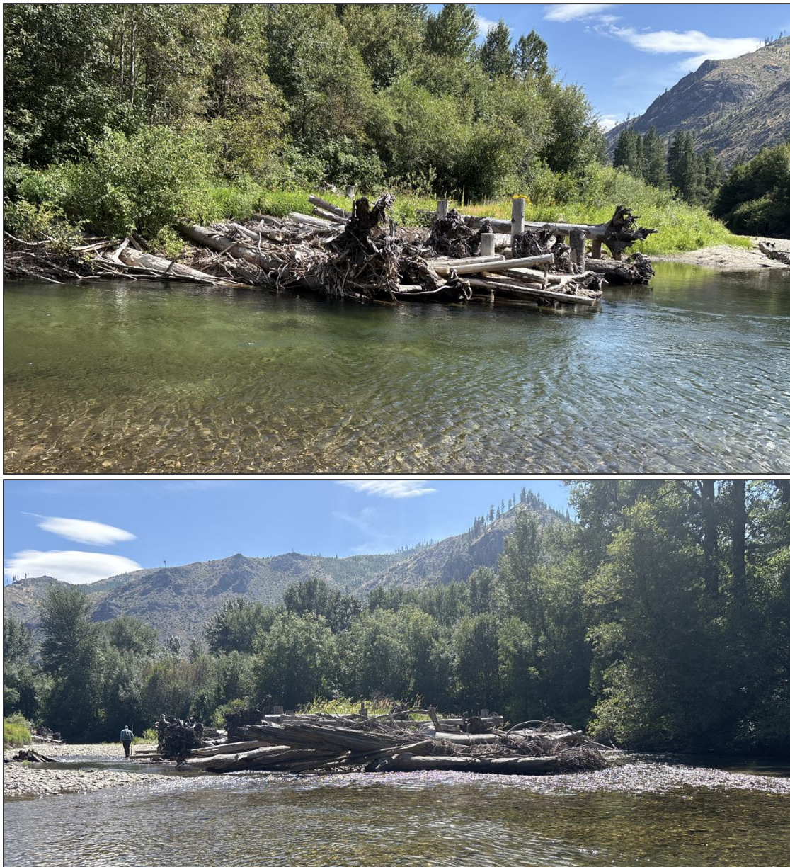
Figure 51. Representative photographs of Stormy C restoration project. Top: Large wood structure on river left at RM 19.5 providing cover to deep pool and deflecting flows into opposite bank. Bottom: constructed apex jam supporting flow split at RM 19.7, looking downstream.
