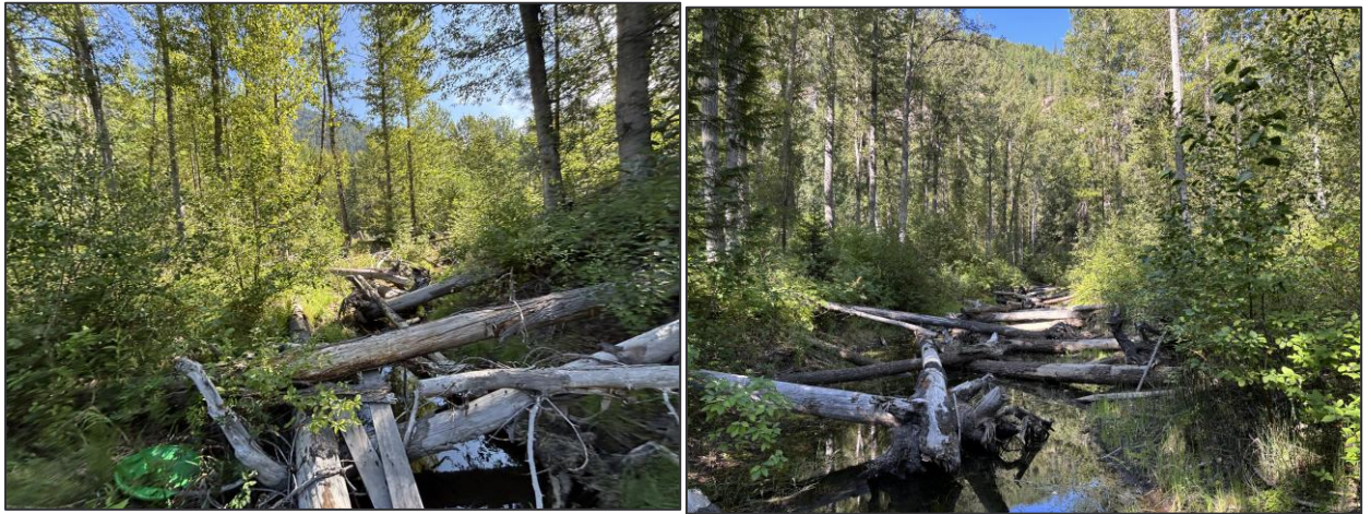
Figure 79. Representative photographs of Entiat 3D restoration project in Segment 4. Top: Large wood structure on river left downstream of RM 26.4. Bottom left: channel with installed large wood for cover, connecting floodplain pond on river right to main channel near RM 26.25. Bottom right: mouth of intermittent river right side channel with added large wood for cover near RM 26.2.
