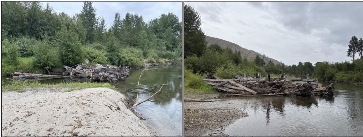
Figure 36. Large wood structures installed during Gray E restoration project near RM 17.8 (left, looking downstream) and RM 17.9 (right, looking downstream).
