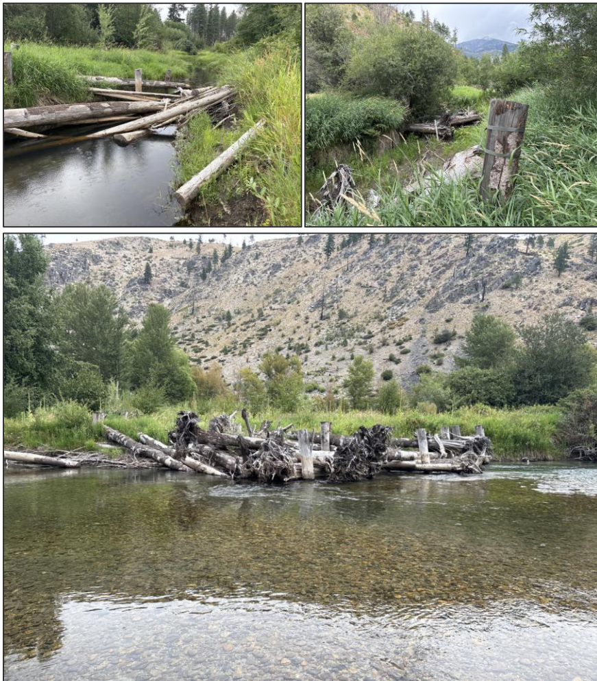
Figure 35. Representative photographs of Gray F restoration project. Top left: wetted side channel through river left side channel downstream of RM 16.8; Top right: dry side channel through river right floodplain near RM 16.85; Bottom: constructed large wood structure on river right near RM 16.8.
