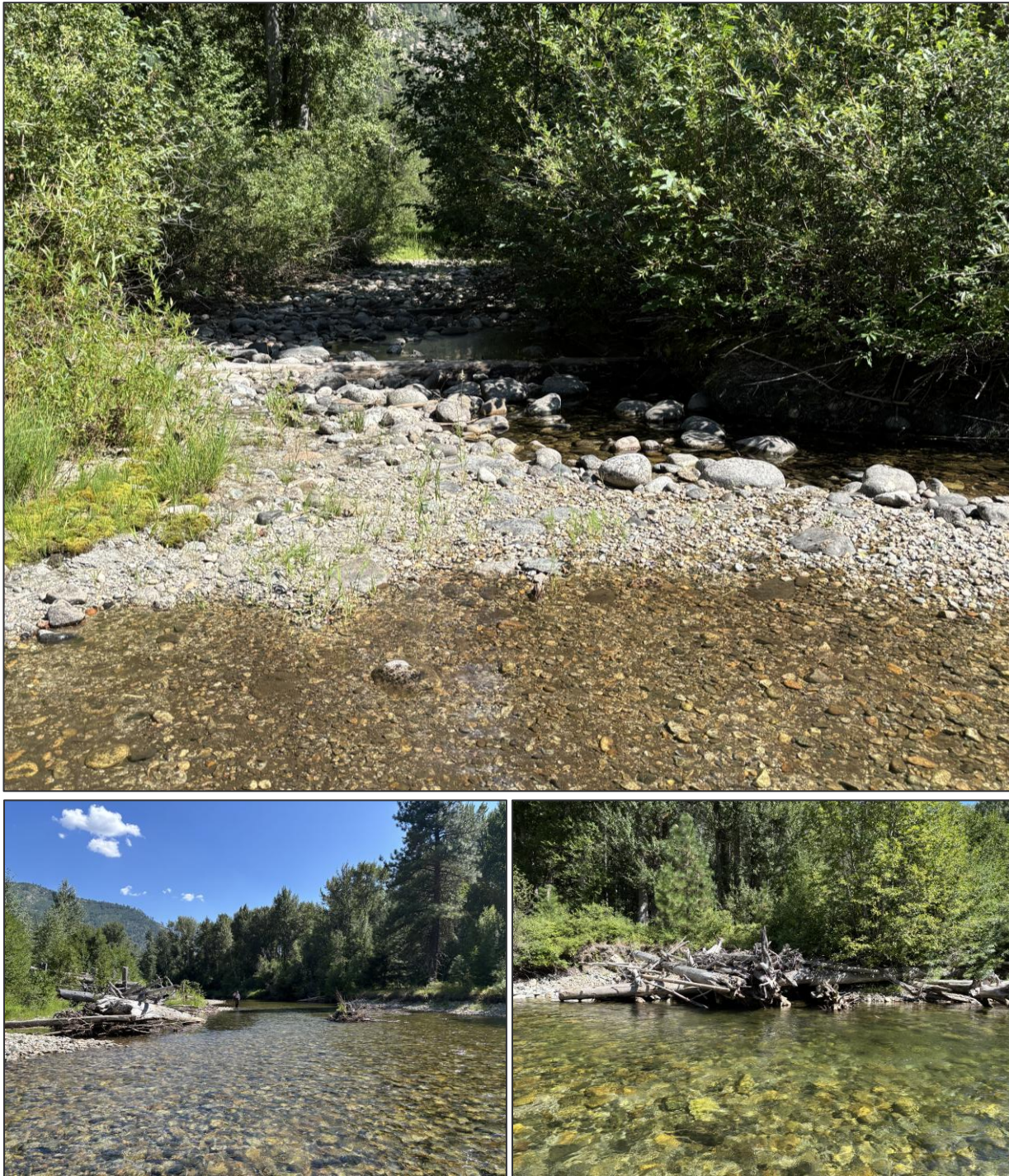
Figure 68. Top: Entrance to side channel reconnected by breaching Upper Tye Levee. Bottom: Constructed large wood structures associated with the Entiat Tye restoration project in Segment 3. Left: looking downstream near RM 23.6. Right: looking toward river left, RM 23.85.
