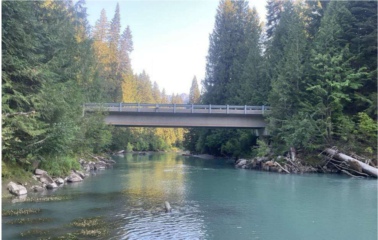
Figure 118. Sears Road bridge and associated bank riprap at RM 7, looking downstream (August 6, 2024).
