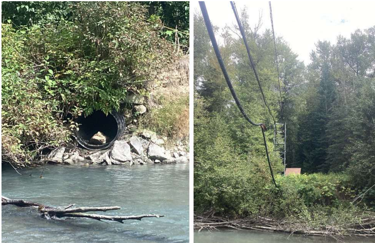
Figure 200. Left: Culvert draining historic channel on river left, entering the Napeequa River at RM 0.1 (September 11, 2024). Right: Cables over Napeequa River at RM 0.17 (September 11, 2024).
