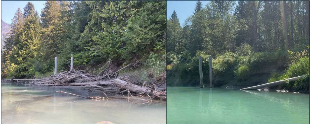
Figure 79. Left: Installed vertical wood pilings with wood accumulation, at RM 3.71 (August 14, 2024). Right: Installed pilings lacking large wood accumulation and retention, at RM 3.92 (August 14, 2024).
