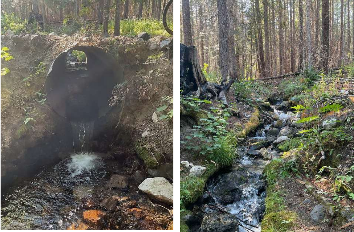
Figure 225. Left: Sears Creek crossing under Sears Creek Road (Forest Road 6404). Right: Sears Creek upstream of the crossing (August 2024).
