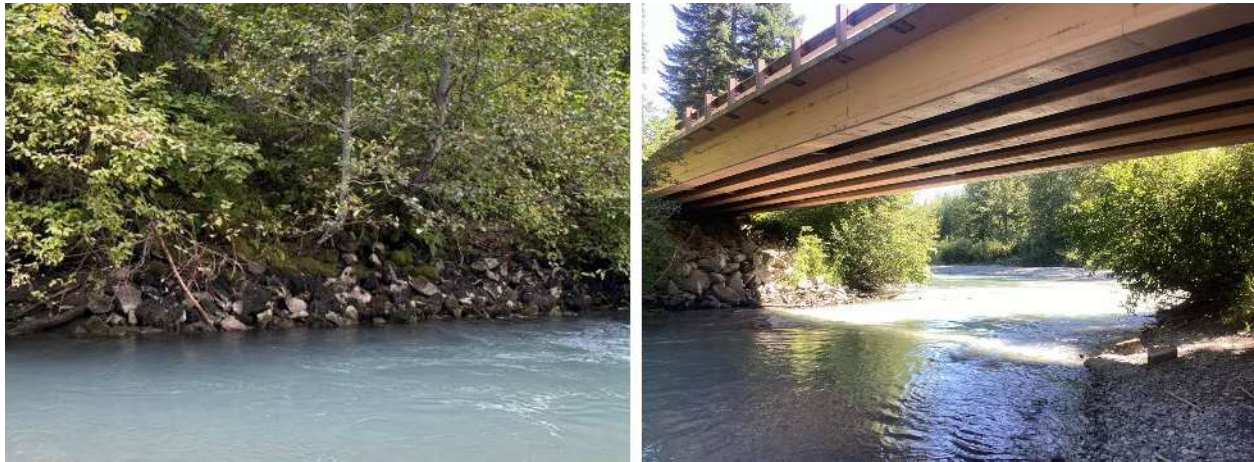
Figure 199. Left: Bank protection (riprap) at RM 0.05 on river-right (September 11, 2024). Right: White River Road bridge over mouth of Napeequa River and associated bank protection (September 3, 2024).
