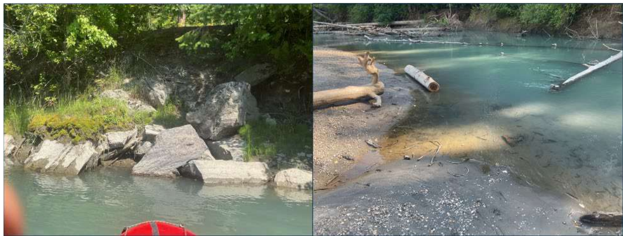
Figure 91. Left: Riprap protecting White River Road on river left at RM 5.43 (August 13, 2024). Right: Sawed off portion of in-stream large wood at RM 5.1 (August 13, 2024).
