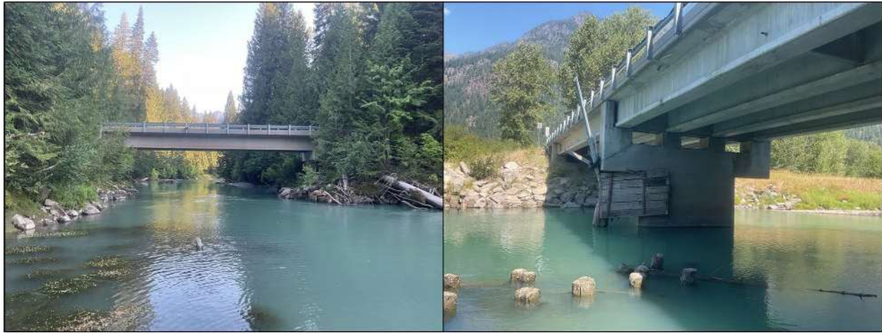
Figure 19. Left: Bridge and riprap over the White River at RM 7 (August 6, 2024). Right: Bridge and riprap crossing White River at RM 2 (August 15, 2024).
