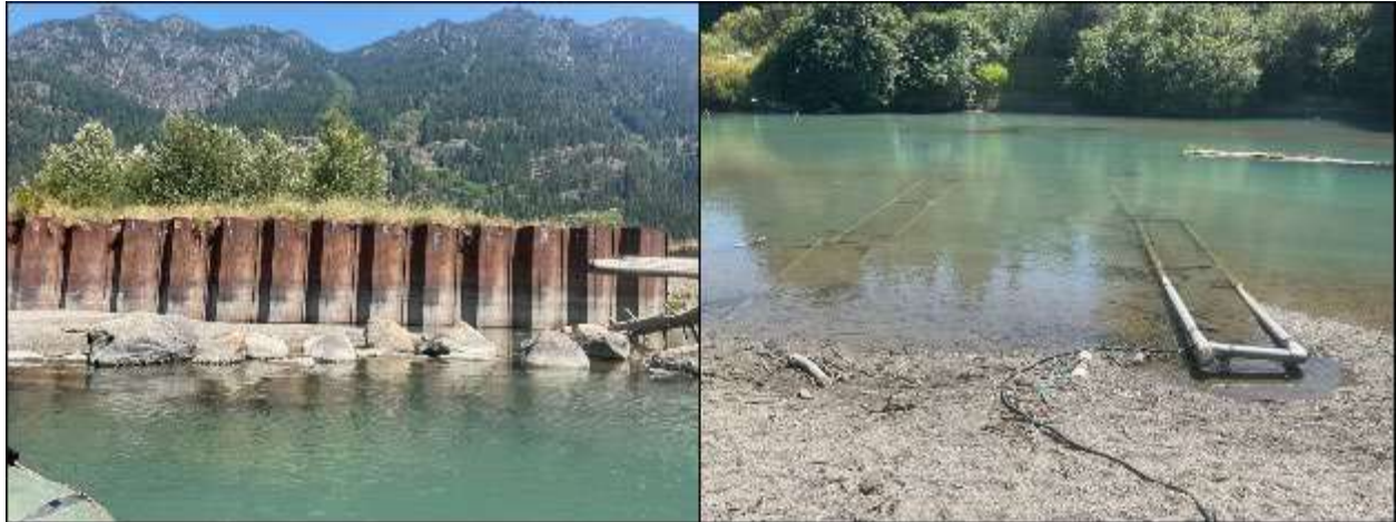
Figure 59. Left: Sheet piles and riprap protect the river left bank from ~RM 1.94-2. (August 15, 2024). Right: PIT tag readers installed on river left at RM 1.8 (August 15, 2024).
