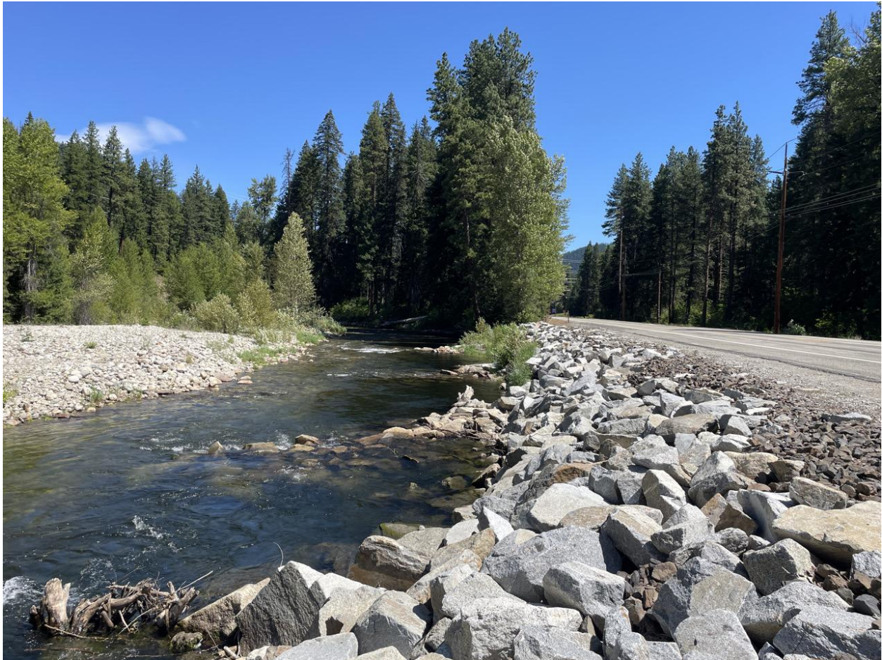
Figure 48. View downstream at bank armor along State Route 207 near RM 4.4 (Inter-Fluve photo July 2005).
