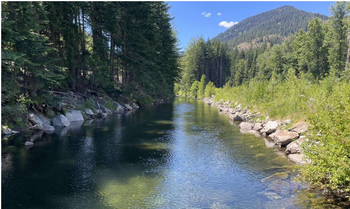
Figure 136. View looking upstream near RM 13 showing riprap along both sides of the channel. This is the historically relocated and ditched channel segment. The railroad is on the left. The right side is just upstream of the prior UWP (upper) project where a levee was removed and riparian/floodplain revegetated, but riprap was left in place (Inter-Fluve photo June 2025).
