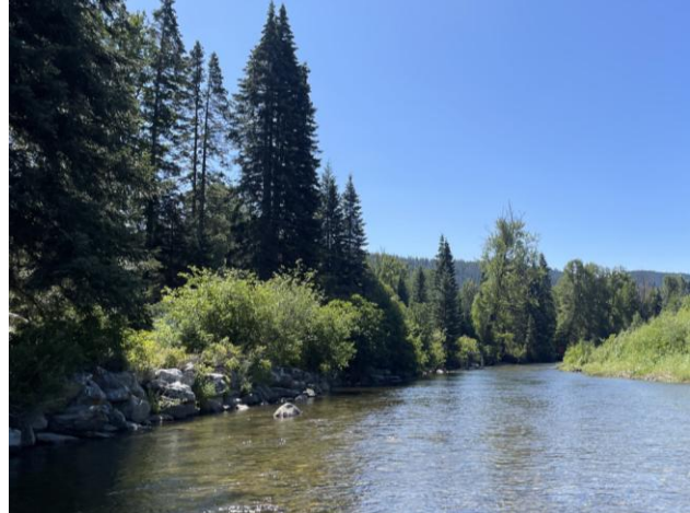
Figure 26. View upstream near RM 0.2 at simplified channel and bank armor on the river-right bank.
