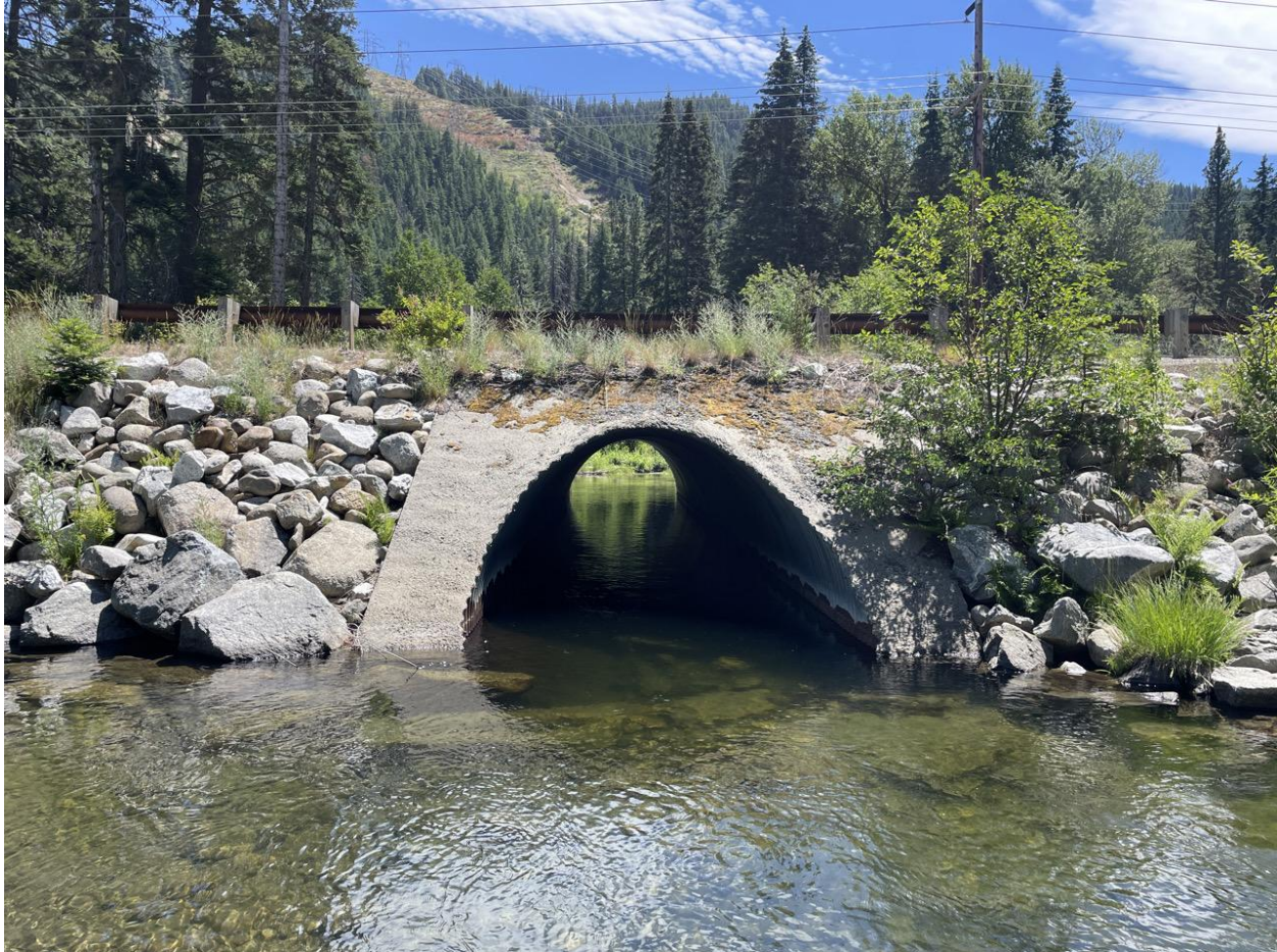
Figure 64. View of culvert under State Route 207 near RM 3.75 (inlet to reconnected ‘oxbow’ side-channel).
