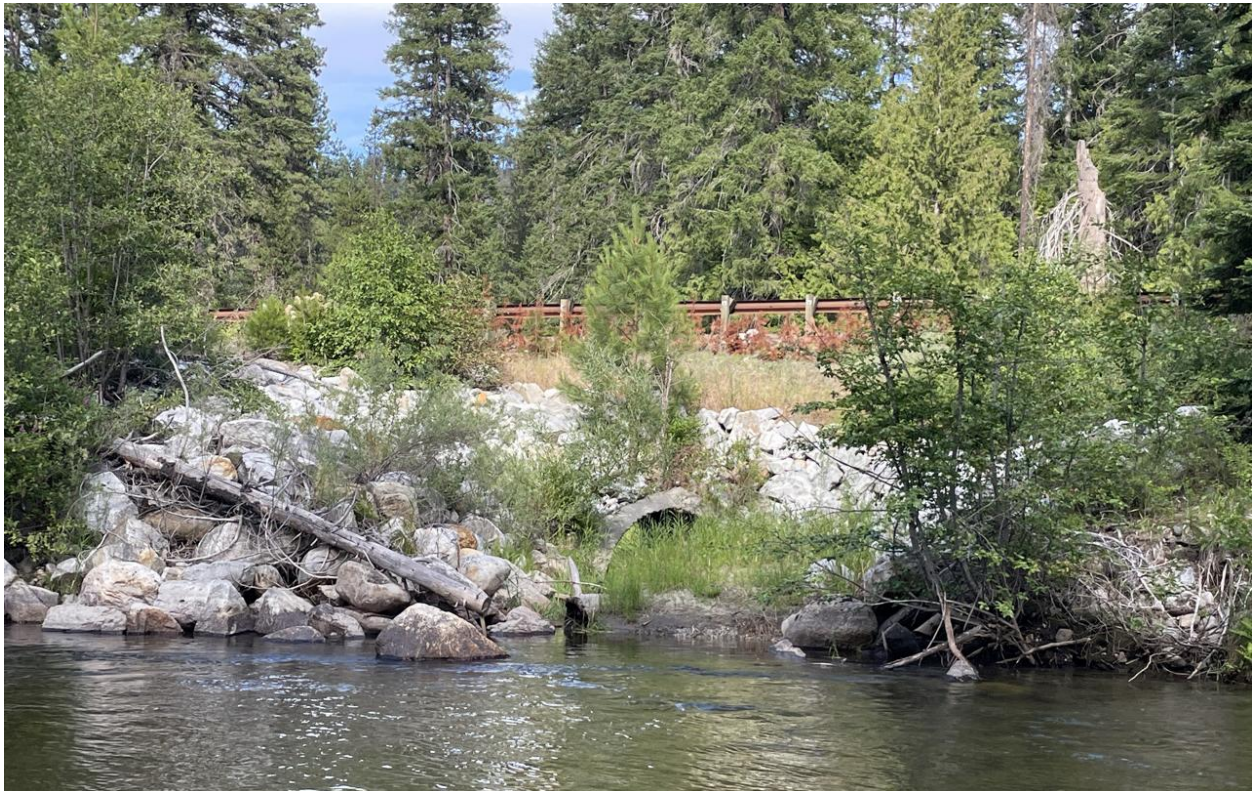
Figure 24. View of river-right bank near RM 1.3 at historical channel cutoff point that is now connected via a culvert under State Route 207.
