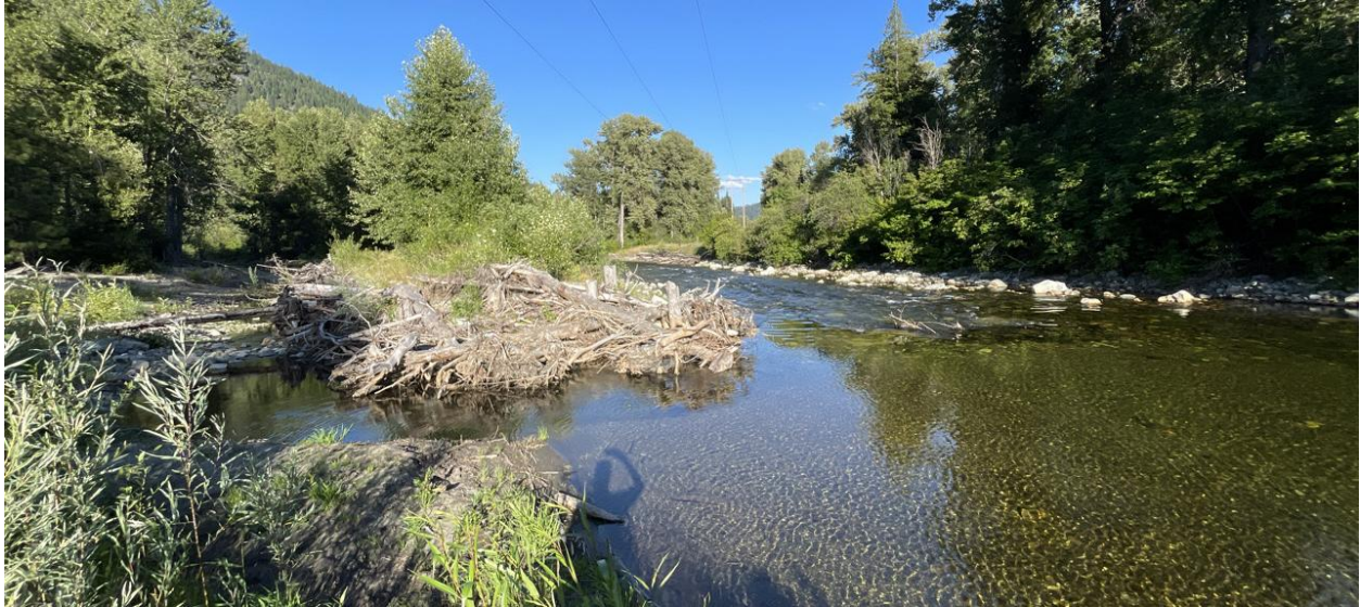
Figure 128. View downstream near RM 10.9 of constructed side-channel inlet (river-left) and constructed riffle (in main channel) at the Merritt Oxbow Reconnection Project (Inter-Fluve photo June 2025).
