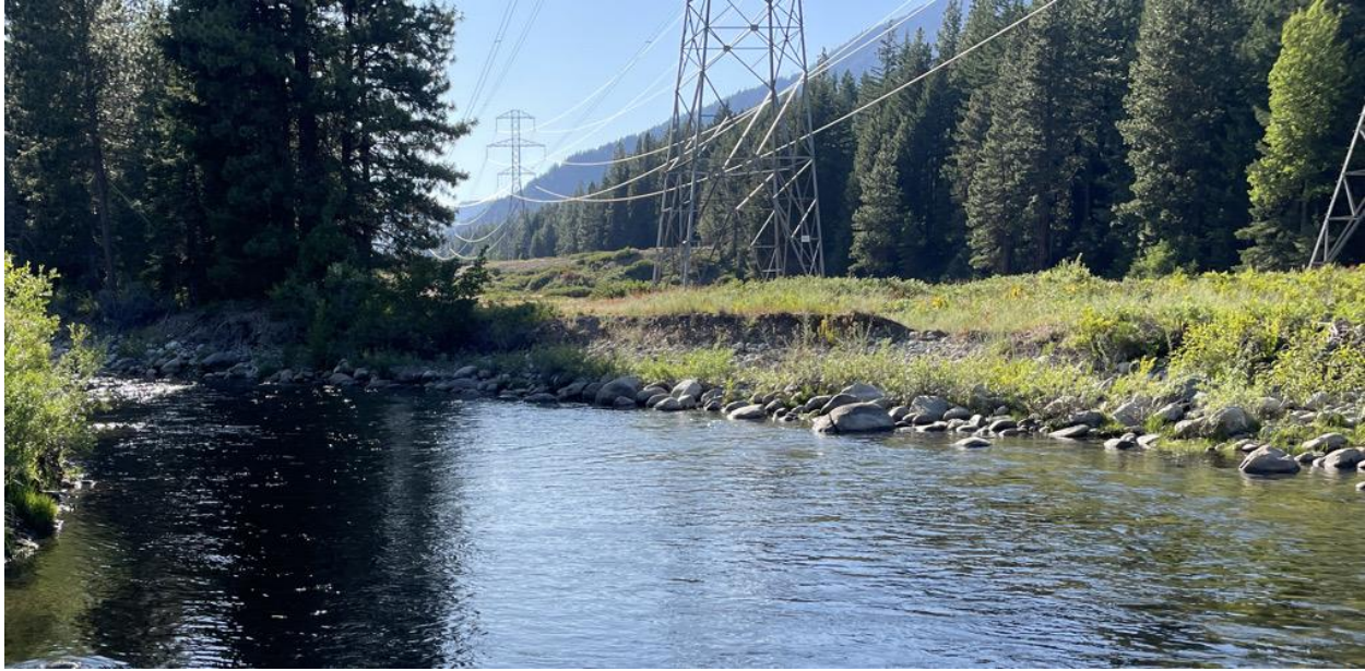
Figure 74. View upstream near RM 5.95 showing bank erosion on river-left bank.
