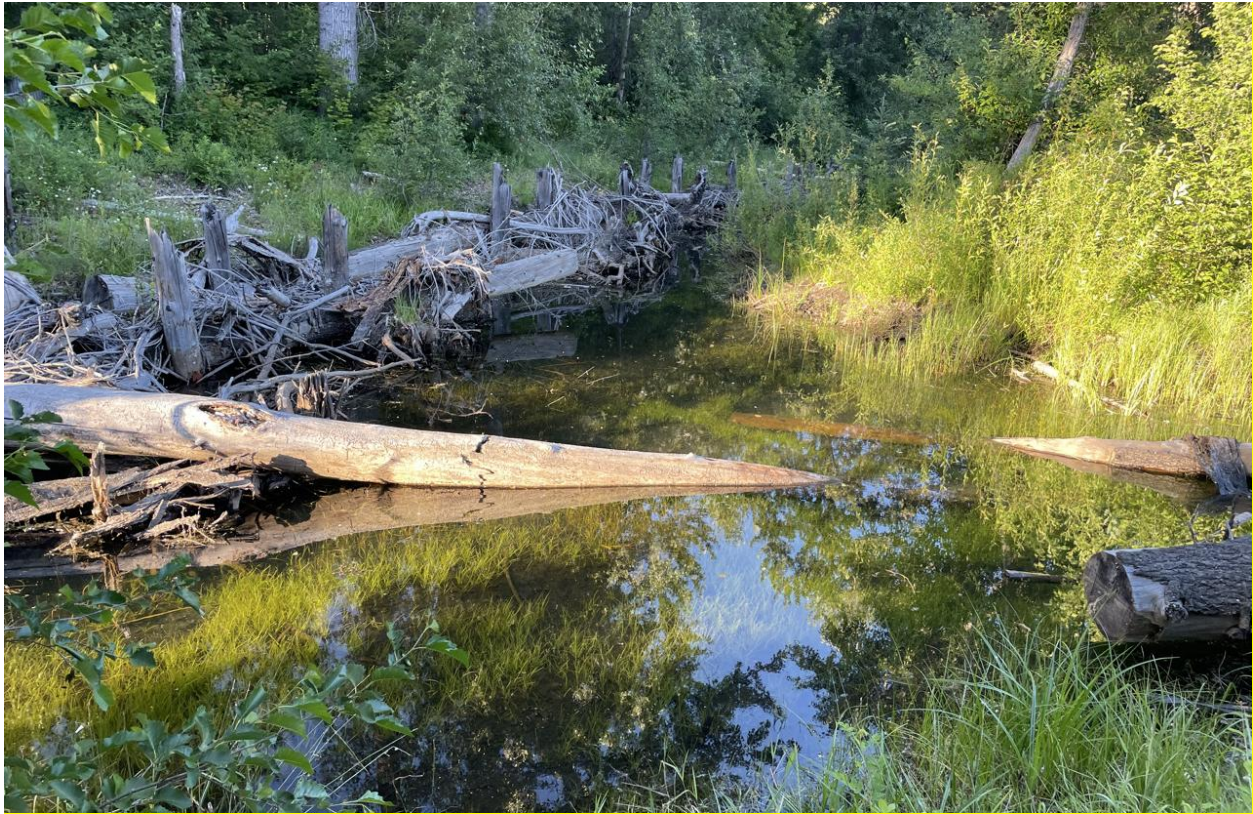
Figure 130. Constructed backwater alcove in river-left floodplain as part of LWP Groups 2&3 Project near RM 10.15 (Inter-Fluve photo June 2025).
