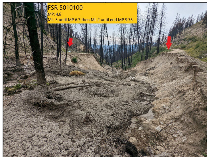
Figure 3.8.4. Post-Cub Creek 2 Fire debris flow and road washout, Butte Creek. Photo credit: Methow Ranger District.
