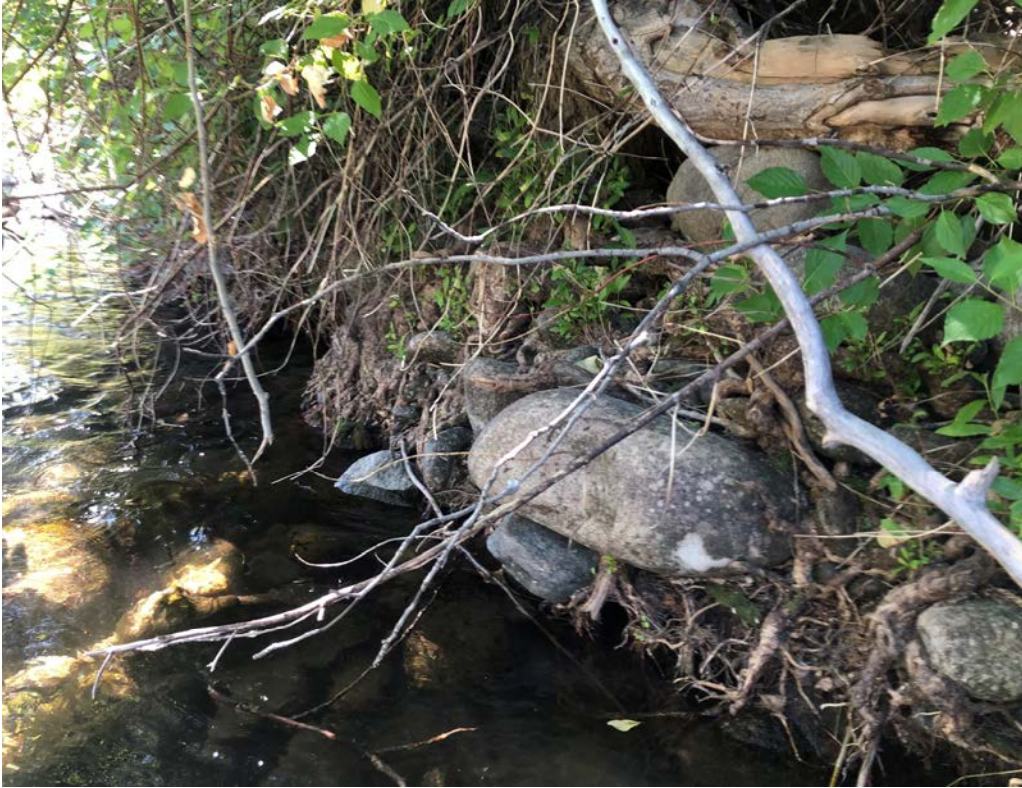
Figure 5: Typical bank armoring with coarse cobble and root cohesion.
