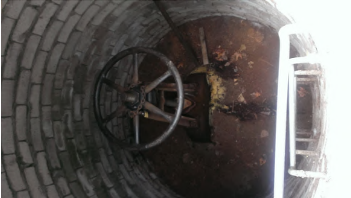
Photograph 5 Inside Valve Enclosure
