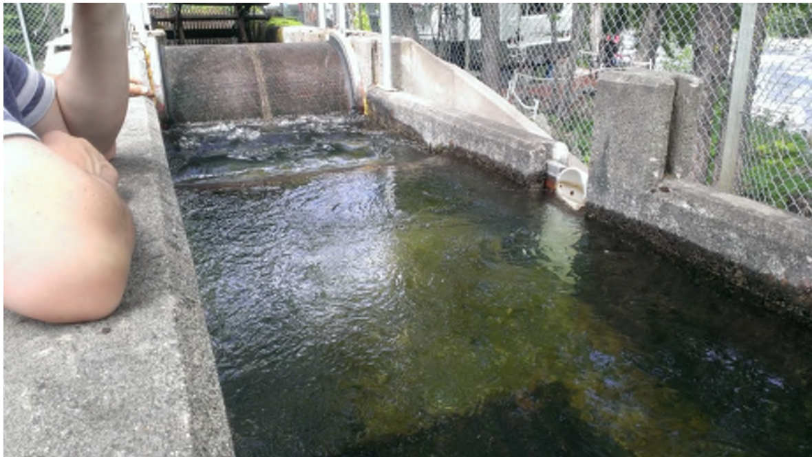
Photograph 6 Bifurcation with Fish Bypass Pipe and Fish Screen
