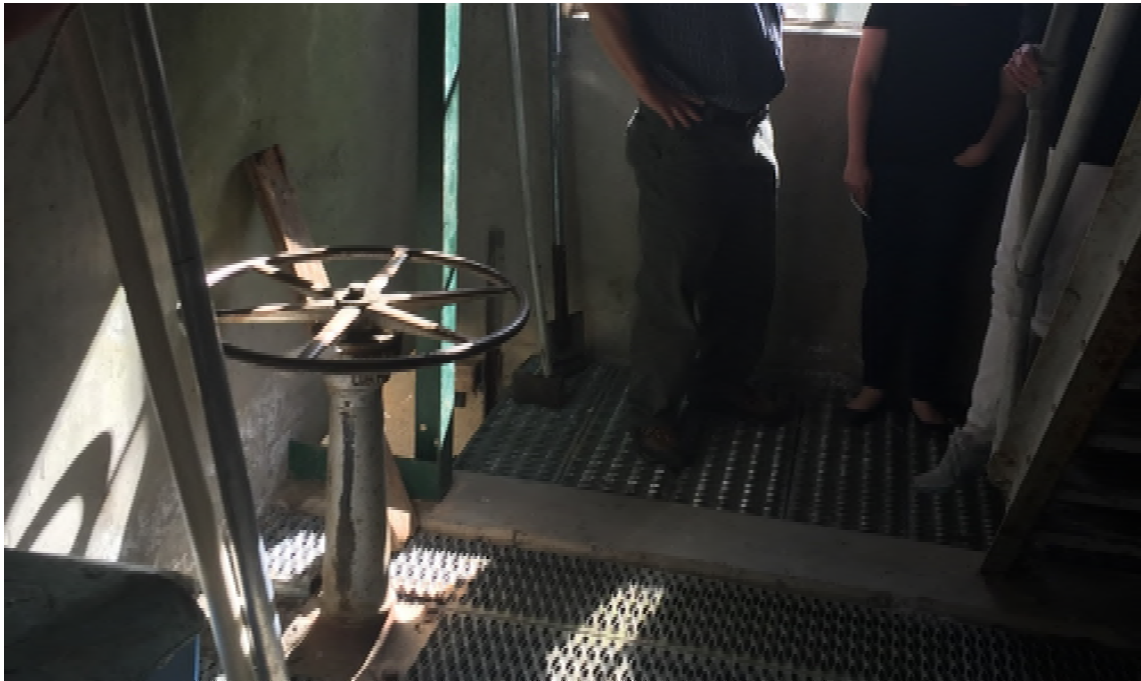
Photograph 3 Inside Control House with Control Gate Operator
