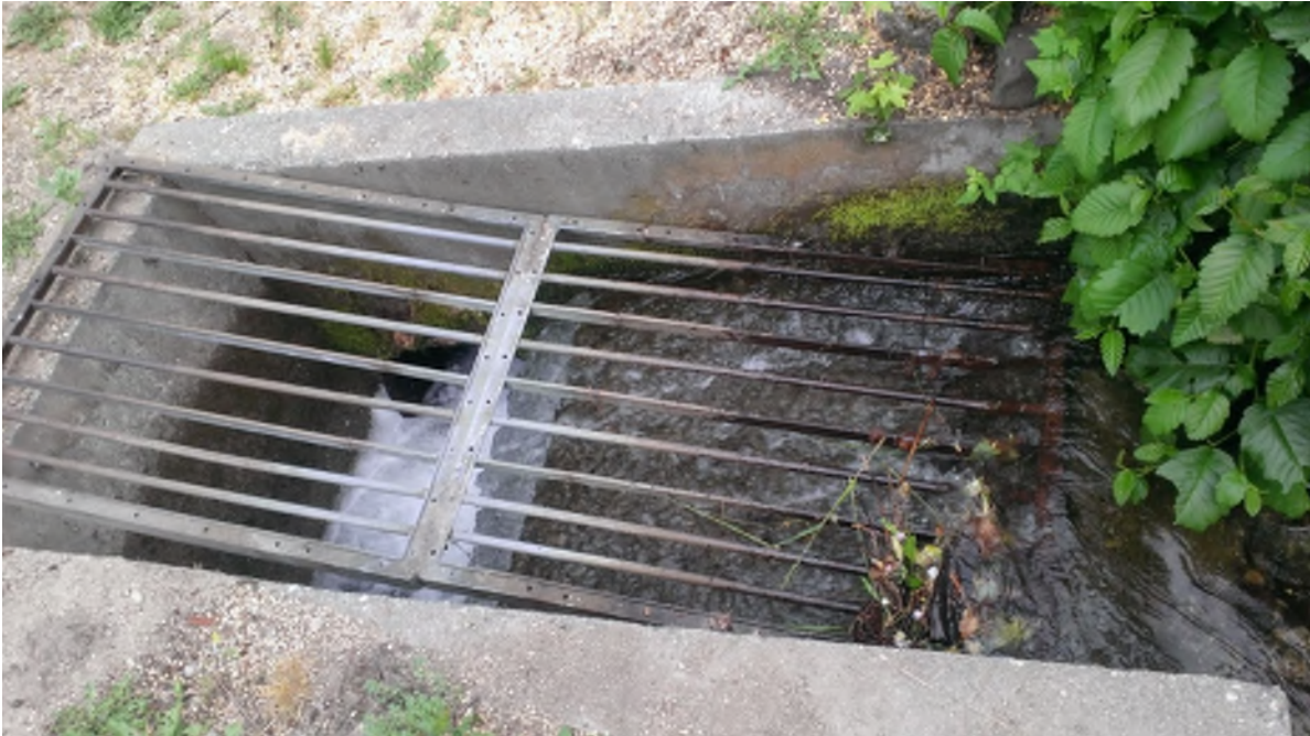
Photograph 19 Inlet to Tailwater Pipeline
