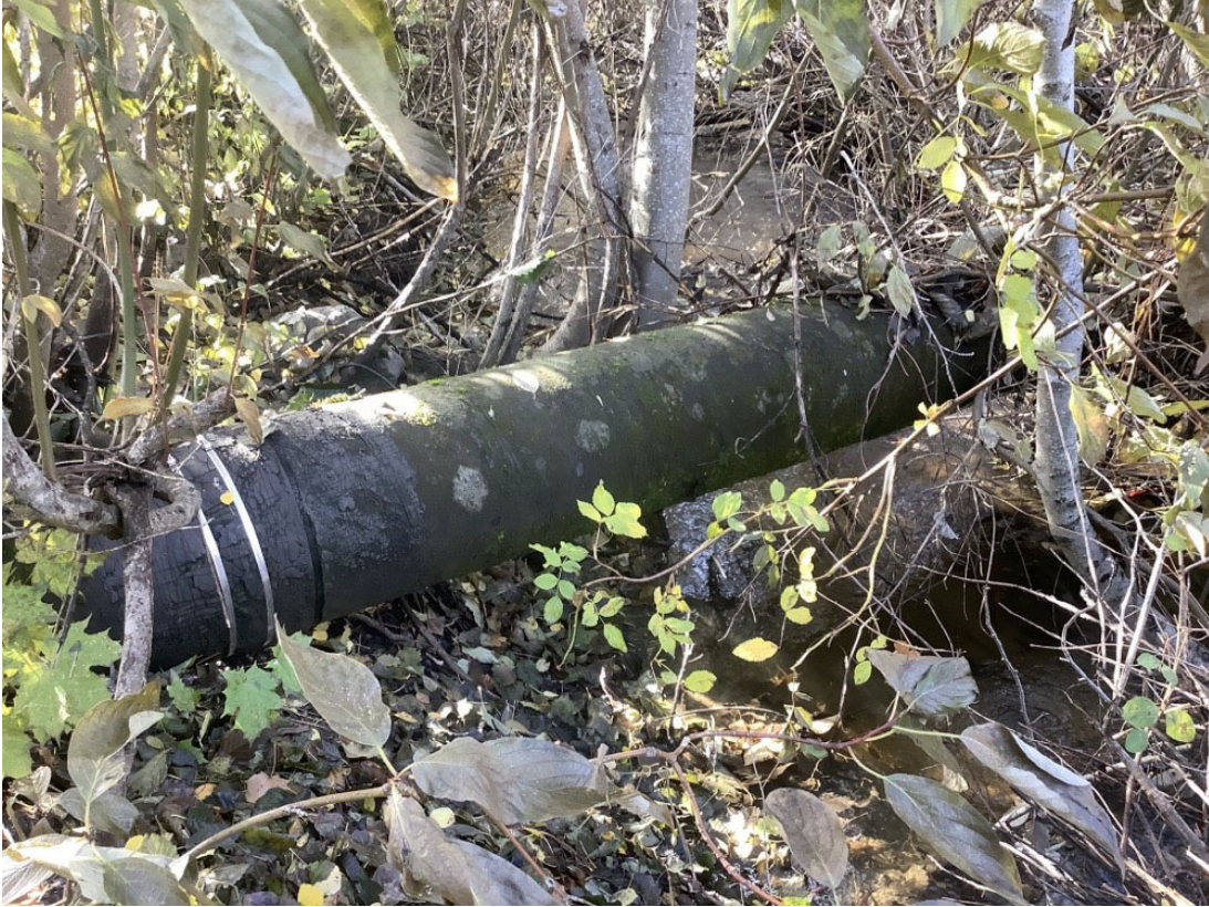
Photo 8. Existing irrigation pipe which crosses Beaver Creek above channel downstream of existing culvert.
